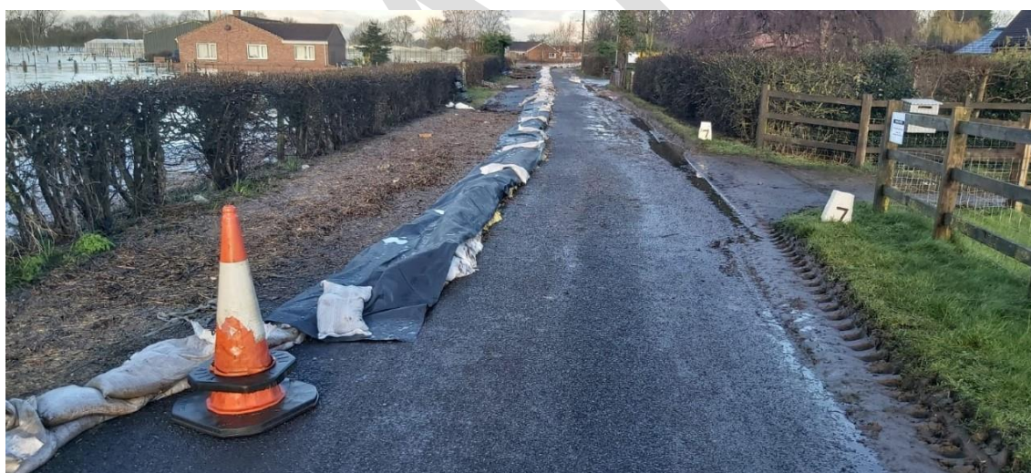
Figure 19: West Bank Visqueen and Rubble Defence
