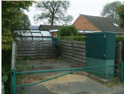
Gas valve house in need of screening
