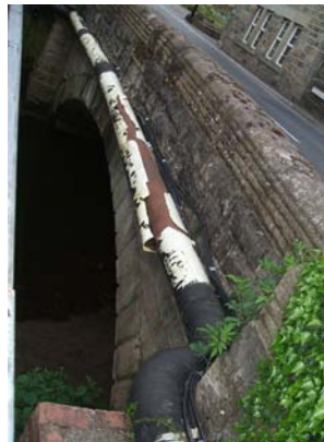
Disfigurement of Pannal Bridge
