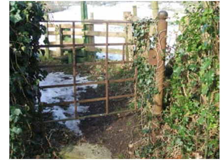
Gate needing repair at Spring Lane
