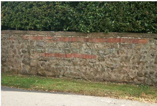
Clock Farm wall is composed of a variety of natural and reused materials.
