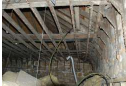
Roof void to NYMR Booking Office showing existing ceiling joists and brackets
