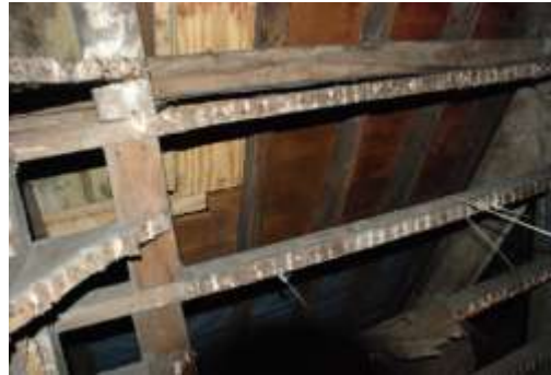
Underside of roof boarding showing patch repairs.
