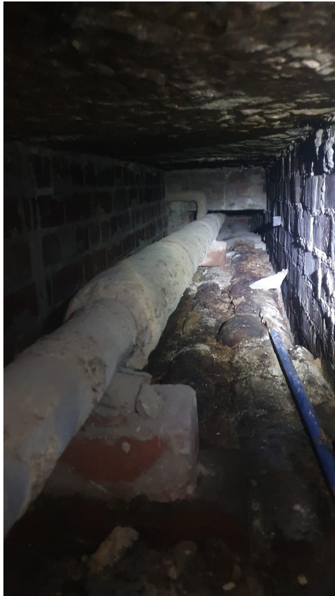
Fig2. Asbestos insulation and buried pipes in duct
